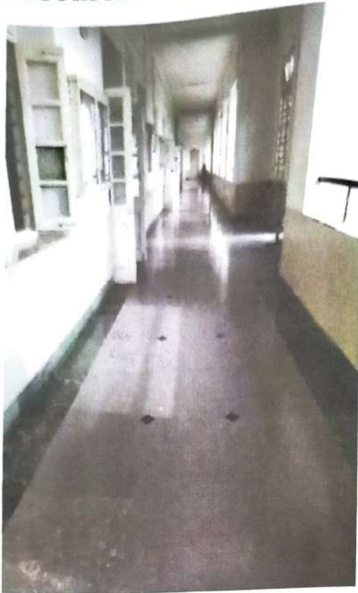
Figure 11 - absence of waste collection bins in the corridor
