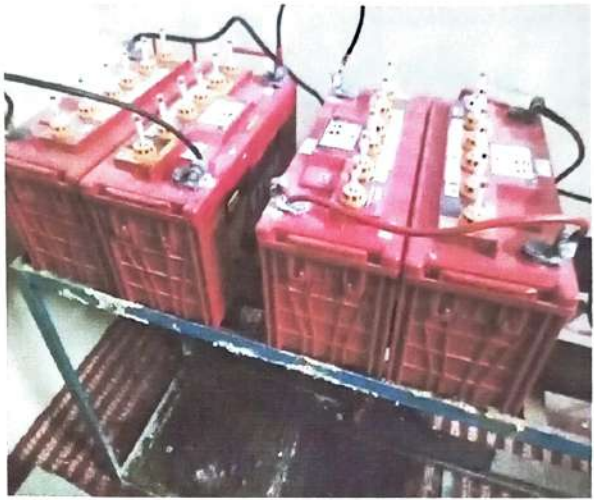
Figure 13 - Placement of battery without ventilation
