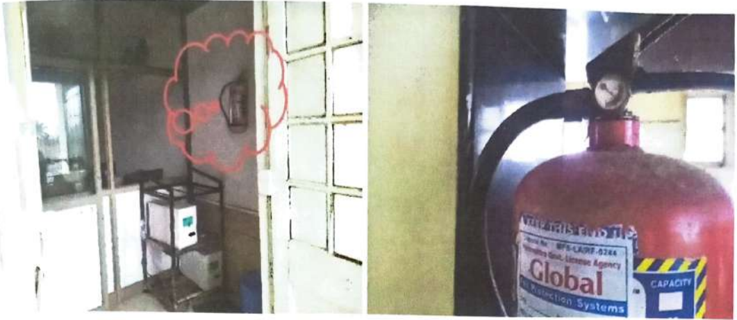
Figure 17 - No ready access to fire extinguisher.
